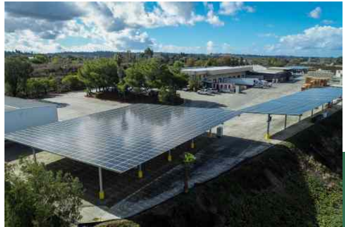
Photo Copyright © Baker Electric
