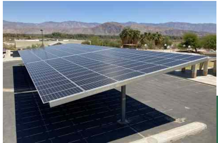
Photo Copyright © Baker Electric
