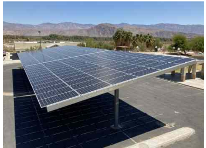
Photo Copyright © Baker Electric
