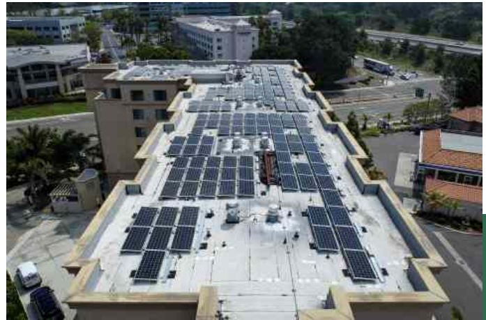
Photo Copyright © Baker Electric
